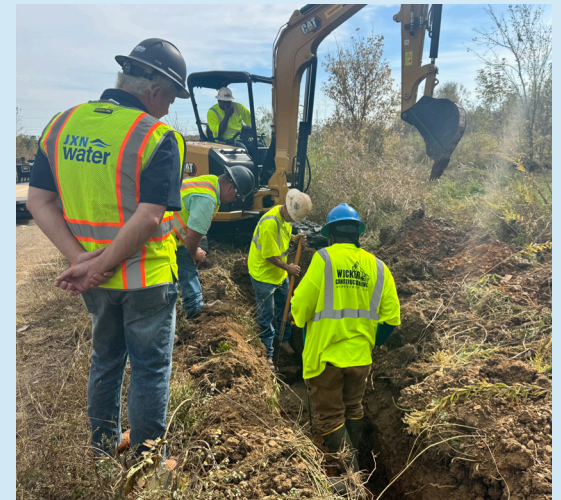
Interim Third Party Manager Ted Henifin oversees work to repair a wastewater leak near a Jackson intersection.
