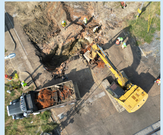
Work is underway near Prentiss and Fortification as crews repair a massive pipe break near and underneath the railroad. The repair is ongoing and will include nearly 100 yards in pipe-replacement in the area.
