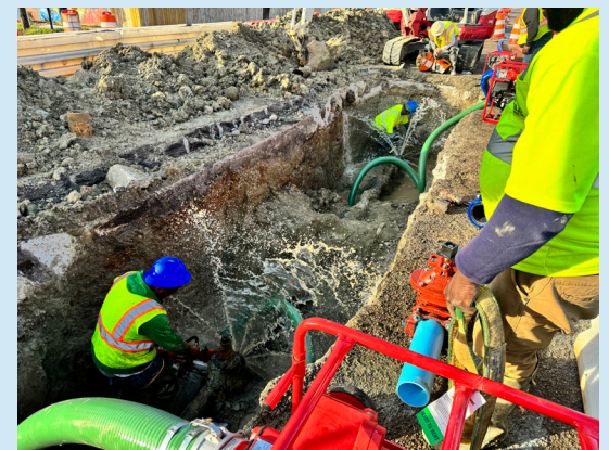
JXN Water crews work on a valve replacement at Fortification and Bailey.
