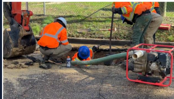
Report: Approx. 98 percent of JXN Water customers now have new water meters
