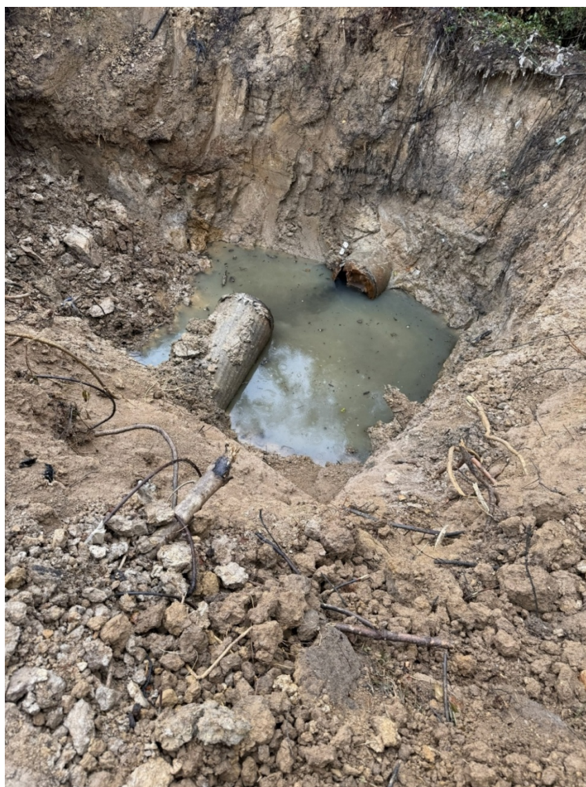
Figure B-1. White Oak (Frontage Road) SSO Photograph
